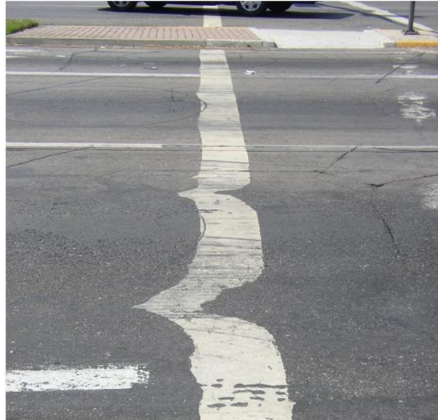
Figura I.C.10.1 Defecto de Combas
